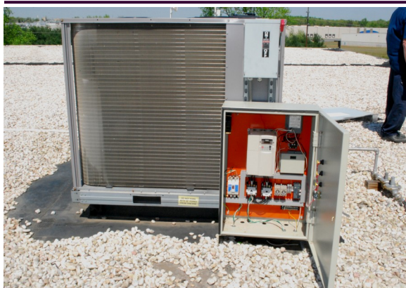
Installation of the H.E.L.P. System onto a standard (Unmodified) "Carrier" HVAC System
